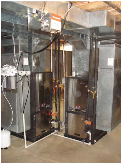
3 & 5 ton open loop geo-thermal systems and RO water treatment system for two (2) steam humidifiers. Installed in Nov. 2007.
